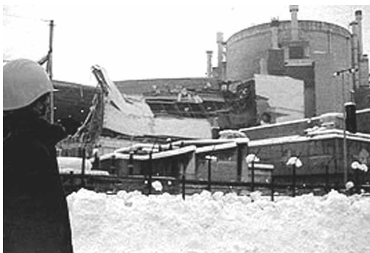
Figure 2.5 Superphénix collapsed turbine hall roof. Photo: Dissident-Media.
